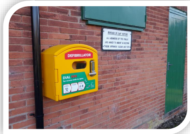
Pictured above: Defibrillator situated on Pavillion building.
