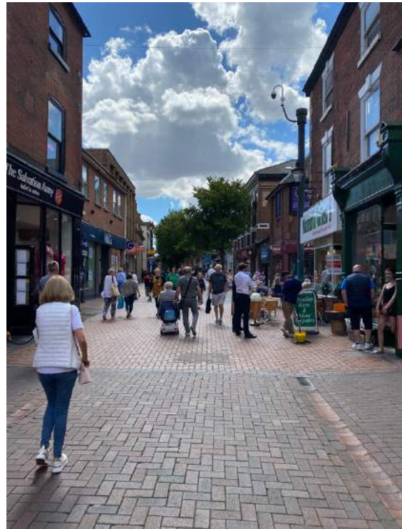
Photo 5 lower quality paving on Carolgate
