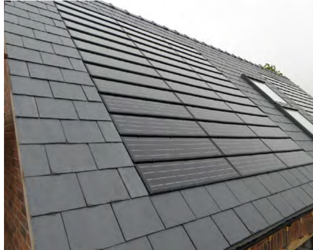
Figure 71: Integrated solar panels on slate roof.
