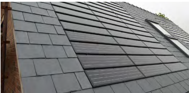
Figure 76: Integrated PV panels on roof
