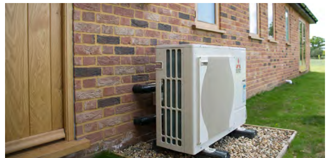
Figure 77: Air heat pump
