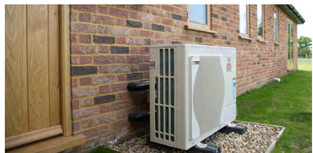
Figure 77: Air heat pump
