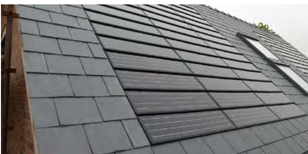
Figure 76: Integrated PV panels on roof
