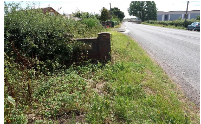
Neglected Boundary, Harworth Road
