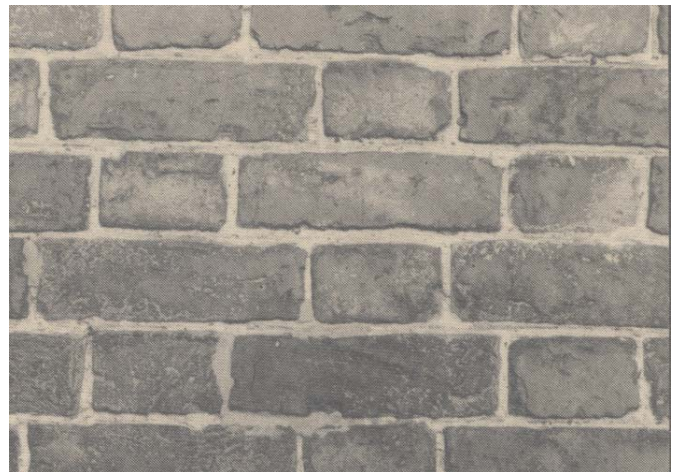
Good repointing of brickwork.
